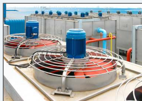
Fans and water pumps
